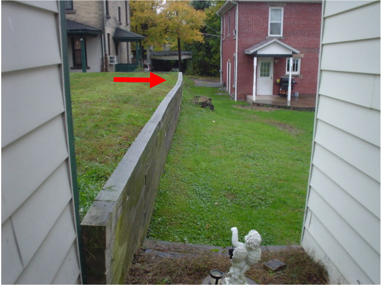
Bulging retaining wall along left side of back yard.
