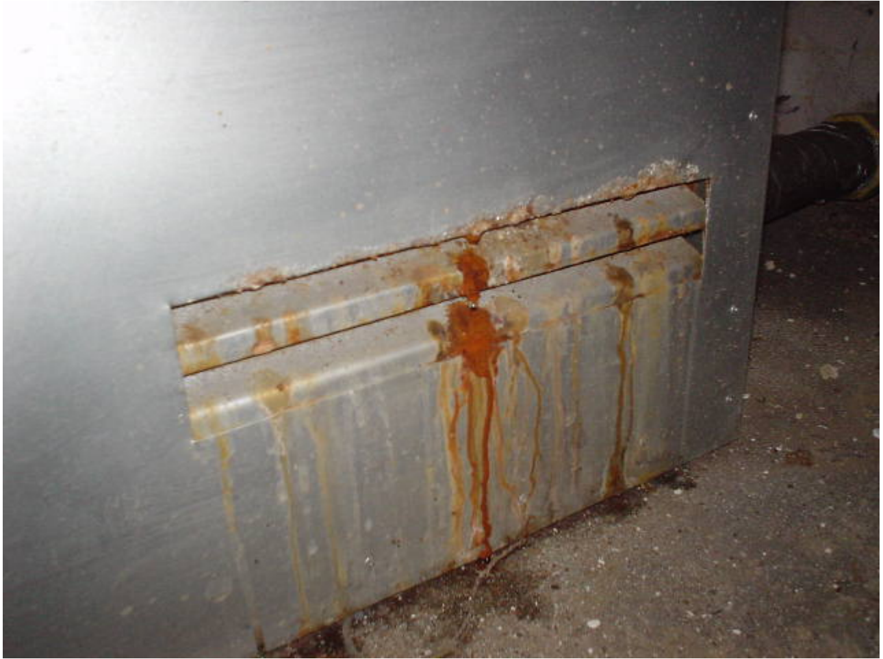
Leak along right side of boiler.
