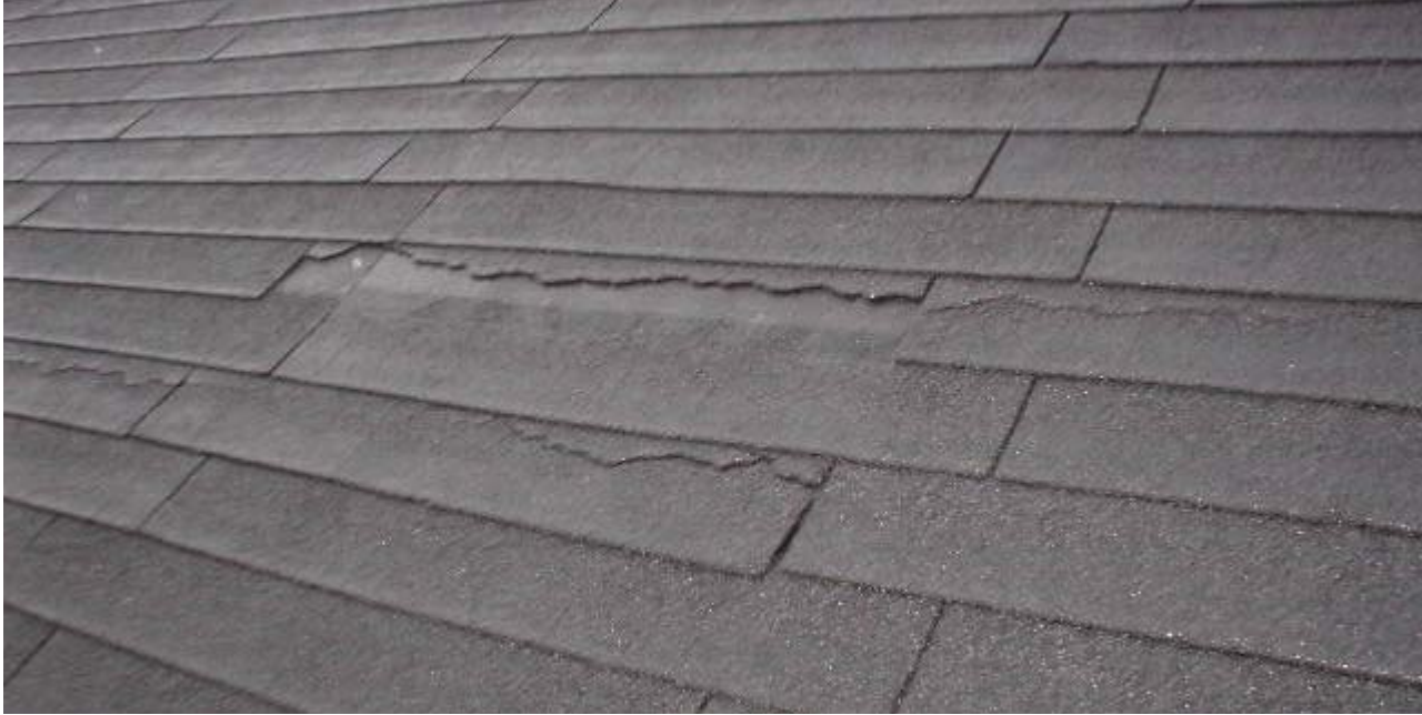
Missing shingle tabs.
