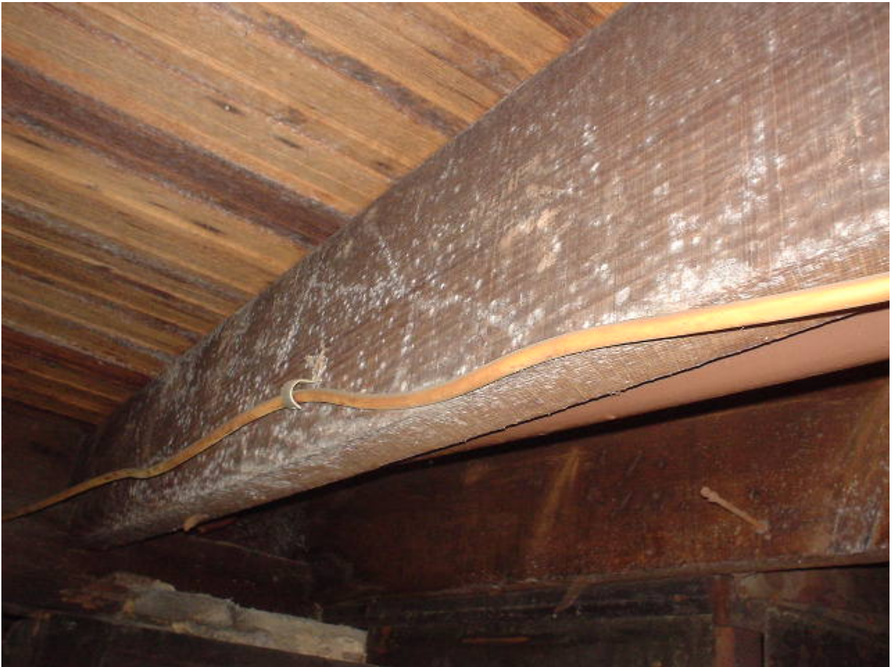
Suspected mold on basement ceiling joist.
