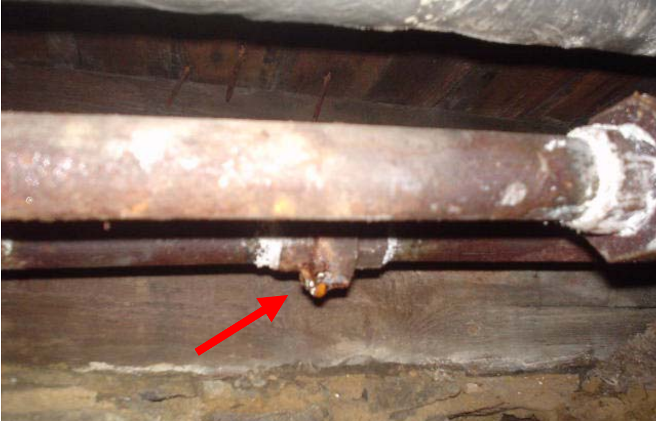
Leak in hot water pipefitting.
