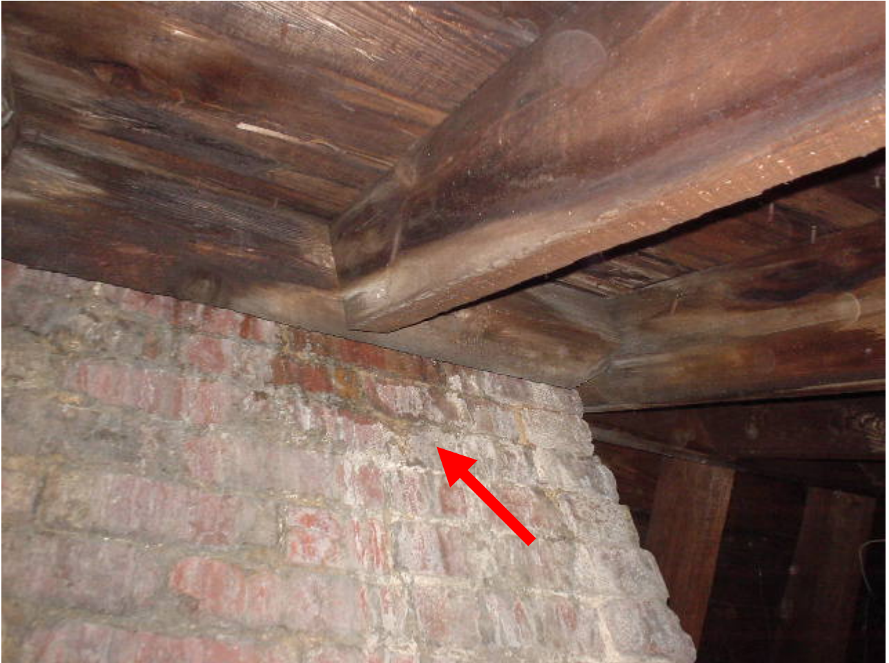
Leak around chimney structure in attic space.
